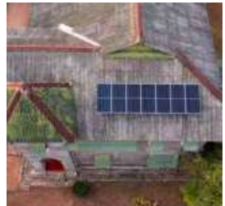
Off Grid Roof Mounted Solar
